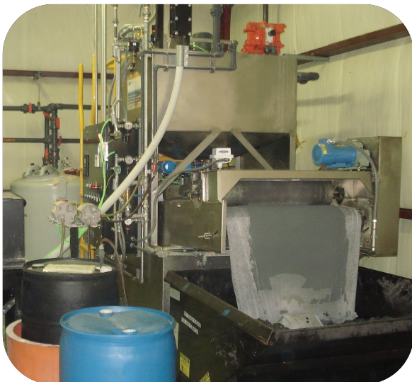
CE-200GA UNIT IN ACTION TREATING ALL PLANT WASTEWATER
