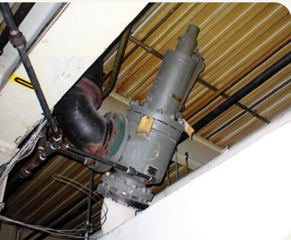
Safety is not installed vertical.
