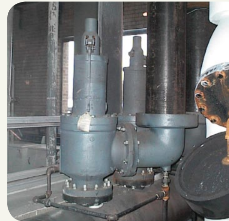
A proper safety valve installation with a drip pan elbow and proper drain lines off the safety valve and drip pan elbow.
