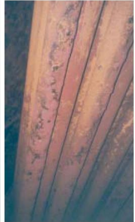
Boiler scaling on boiler tubes in composite boiler
